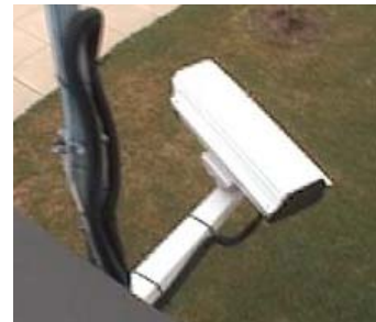
Photo of Weather Station Camera Mounting
